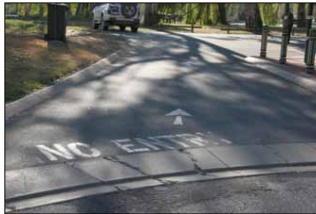
Confusing Pavements Markings
